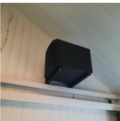
18" sub-woofer fitted using specially TSPProfessional manufactured steel wall brackets
